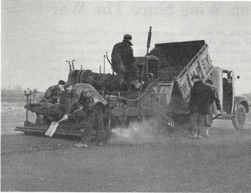
The construction of runways on the South Airfield proceeds steadily, though much remains to be done. Here, one of the machines involved in the work can be seen laying asphalt
