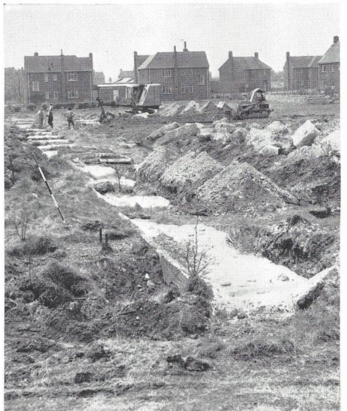
Foundations of the old airship hangars (p. 6) being removed to make way for new married quarters
